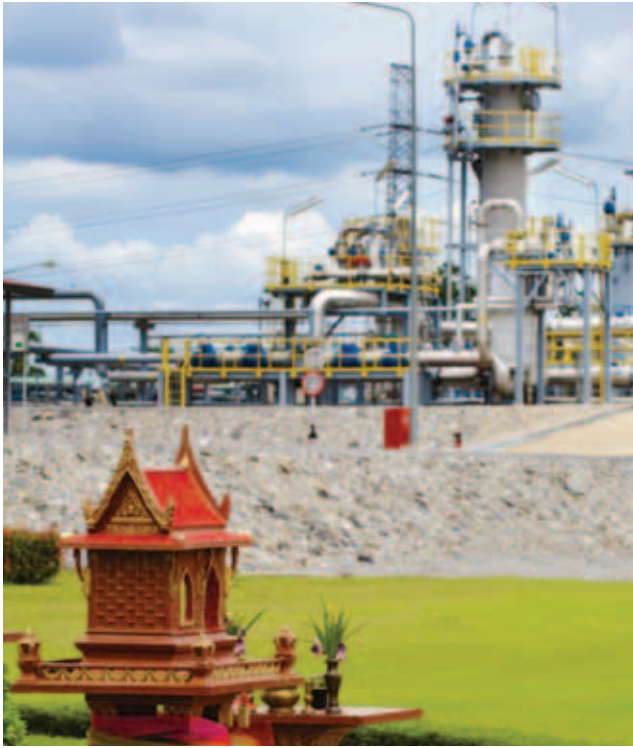
Gas Plant, Sinphuhorm, Thailand
